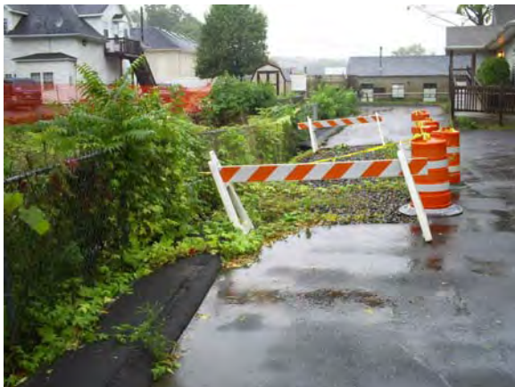
Photo 32: Parking lot undermined at shelter
