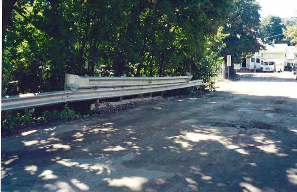
Thorpe Street Extension roadway damage
