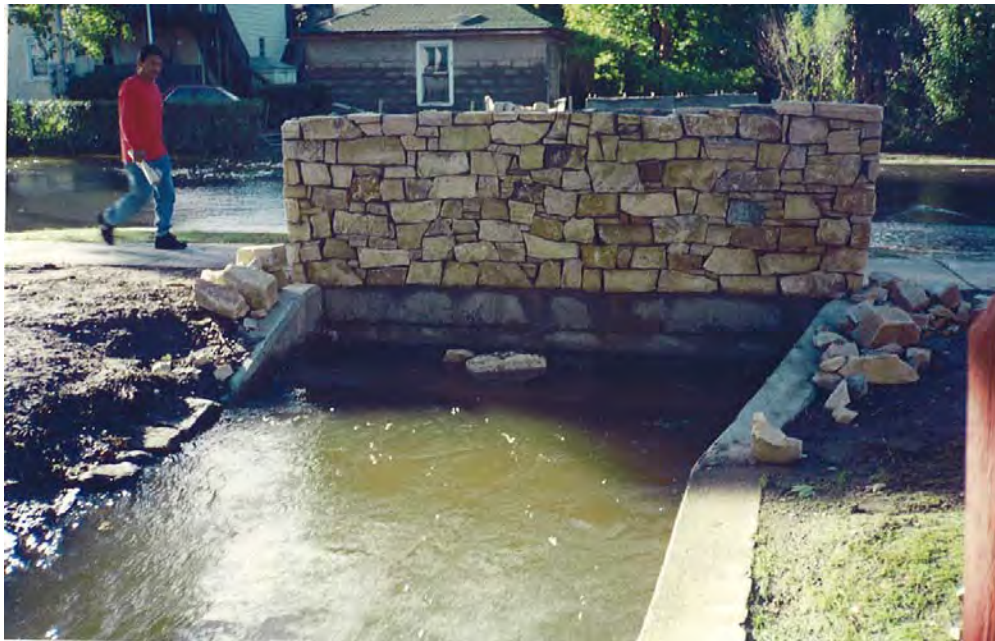
East Pearl Street bridge damage
