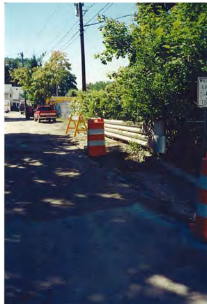
Thorpe Street Extension - Washout
