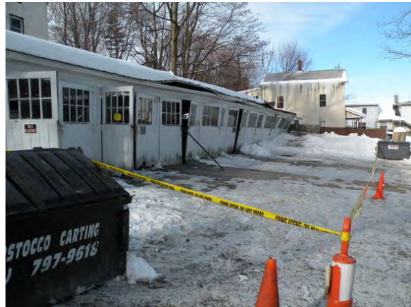
Late January roof collapse of a garage on West Street in Danbury. Photo by Mark Langlois ( http://danbury.patch.com ). Used with permission.
