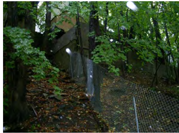
Photo 28: Concrete structure failure above brook
