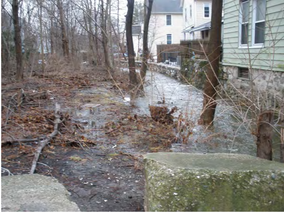
Blind Brook at George Street looking south (upstream). Note culvert wall to right and trees demarking left edge of channel.
