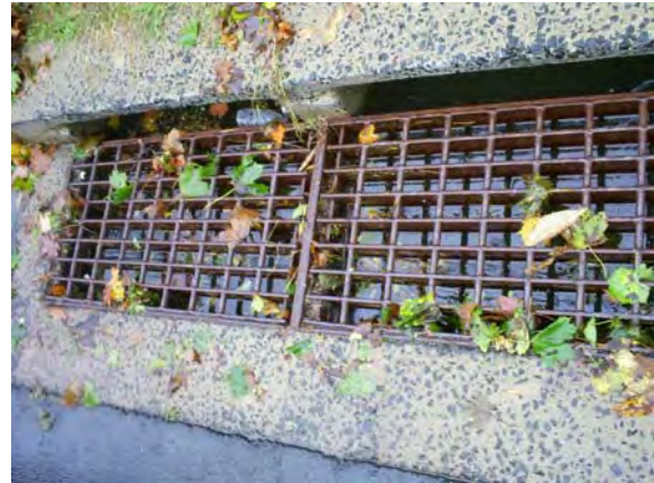
Photo 23: Downstream storm drains full
