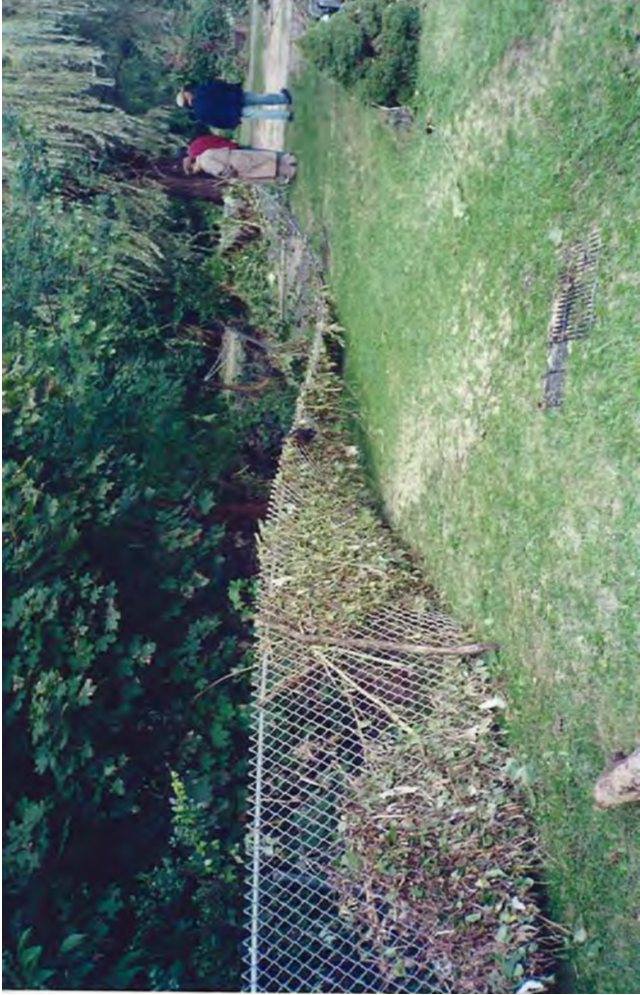
Thorpe Street Extension fence damage
