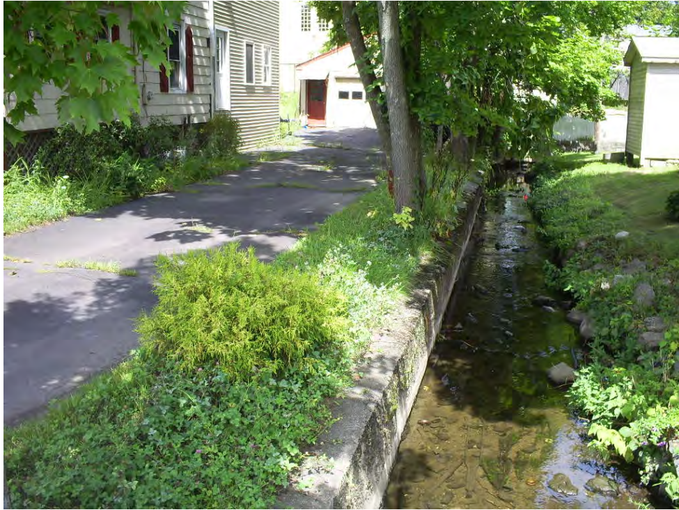
Constricted channel downstream of East Pearl Street bridge over Blind Brook culvert. Repetitive loss property is to left. Note 90-degree turn to right behind shed.
