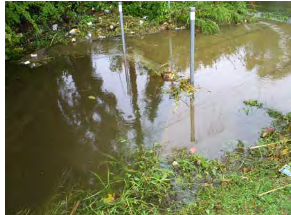
Photo 35: Beginning of Memorial Drive to Overlook Road culvert flooded
