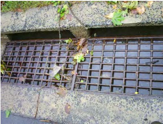
Photo 24: Upstream storm drains full on E. Pearl St.
