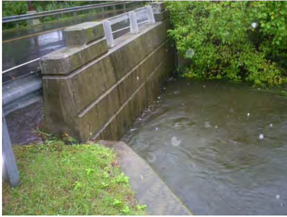
Photo 12: Kissen Brook culvert flooded
