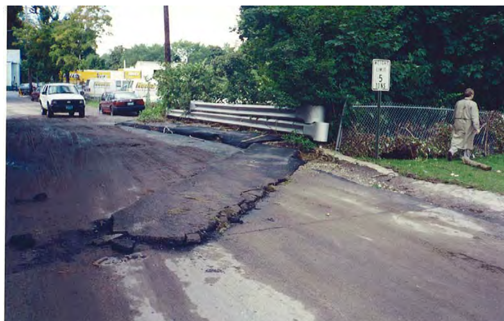
Thorpe Street Extension roadway damage
