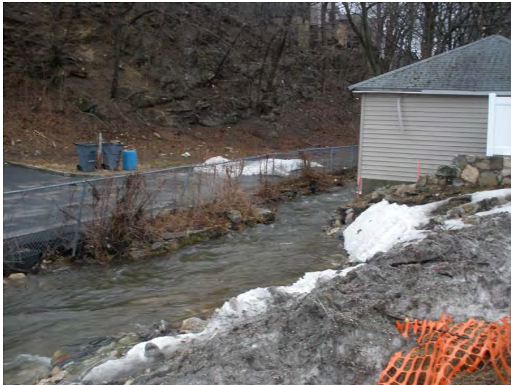
Blind Brook at Pentecostal Church on New Street. Note erosion damage to parking lot in foreground.
