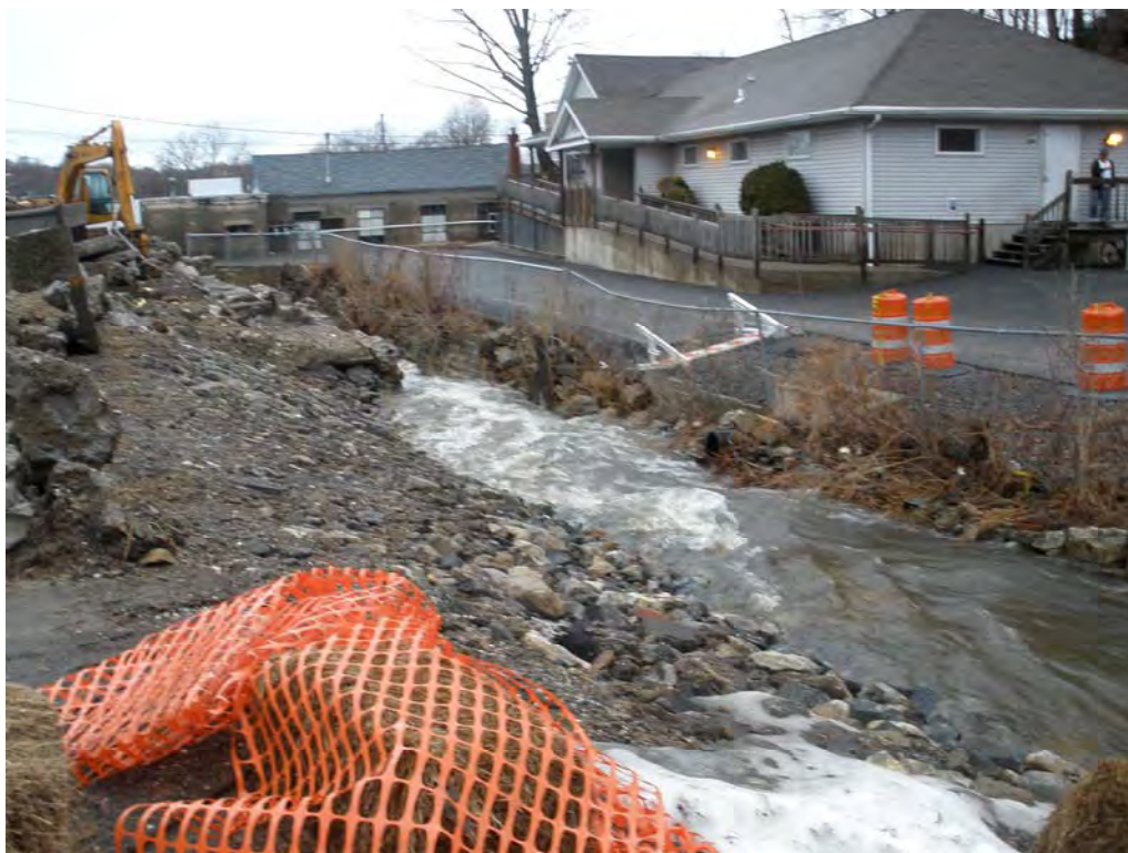
Blind Brook at Pentecostal Church on New Street. Flooding caused major erosion to west bank of stream (church parking lot). Homeless shelter in background.
