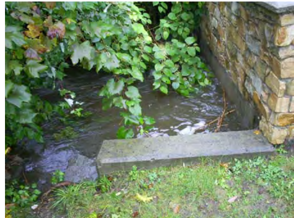
Photo 25: East Pearl St. culvert flooded
