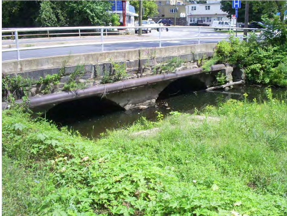
West Avenue bridge over Still River east of railroad tracks, looking downstream from repetitive loss property. Constriction of flow likely exacerbates flooding.
