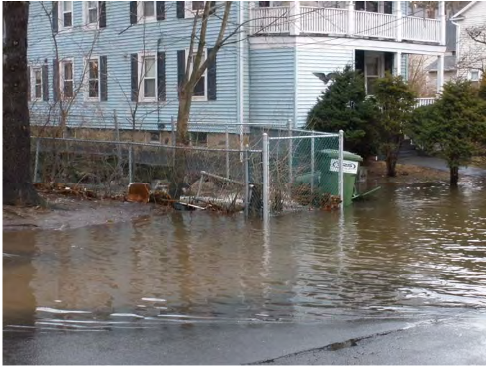
Blind Brook overflowing William Street at exit from William Street culvert near East Pearl Street
