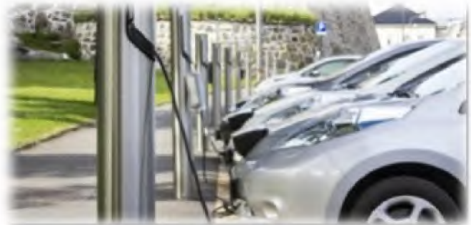
Electric charging stations
