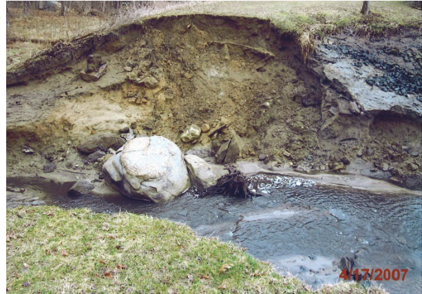
Rogers Pond Dam Breach, April 2007
